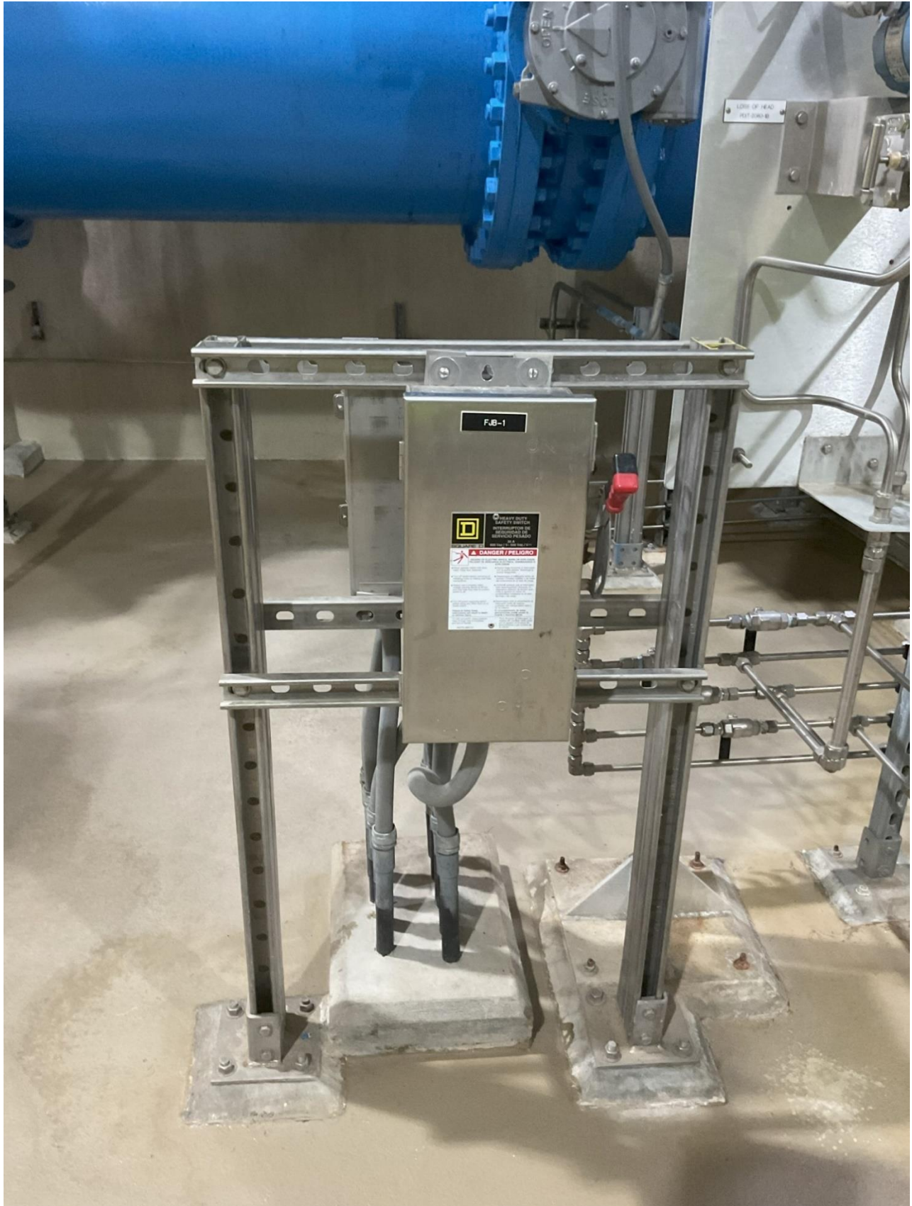
Photo 12: SCFP Existing Power Disconnectf (TYP)
