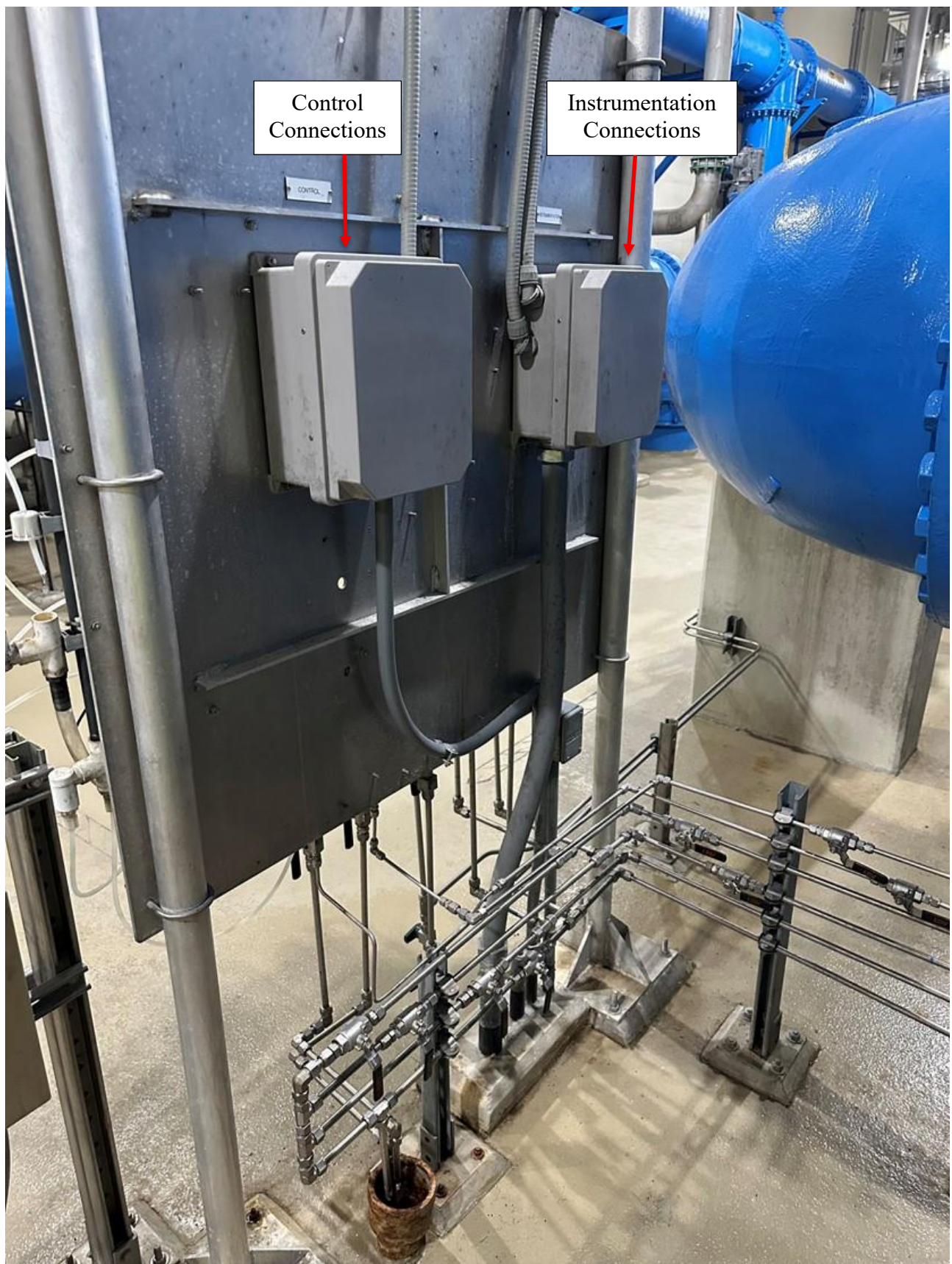
Photo 11: SCFP Existing Control and Communications Connections to Remain (TYP)
